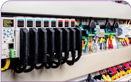
VFD & PLC Panels
