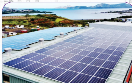
Industrial Solar Installations
